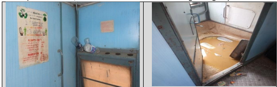
Fig 6: Water Bottles were used by Passengers and kept on window in Train No. 82652 (SWR)
