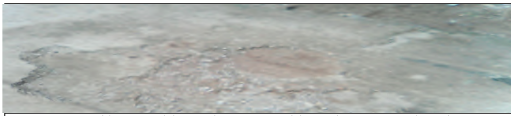
CC road from Mangilal Suman house to Tejsingh house Thungani (GP, Sakrawada)
