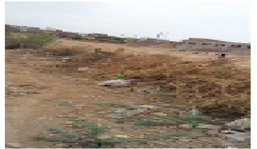
Construction of boundary wall around the sports ground, Jain Public Sanstha at Ganashar road, Bikaner
