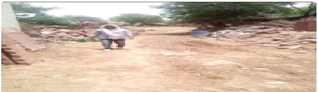
CC road from Dodipura to Mircholi Pura, Jatav Basti damaged at various places
