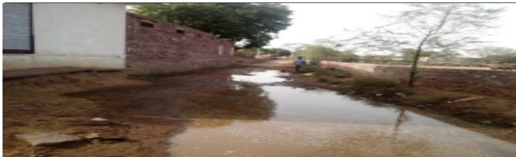
CC road from Ramniwas house to Surendra house damaged at various places
