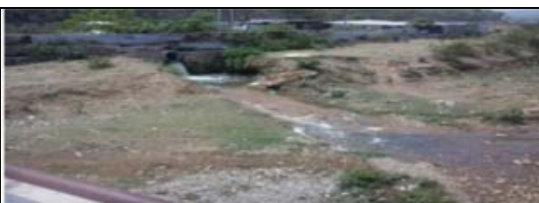
Picture No 2: Disposal of treated effluent in Nalla at Mothorowala
